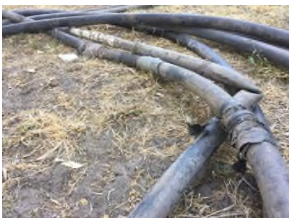
Old water pipe that had been partially "mended"
